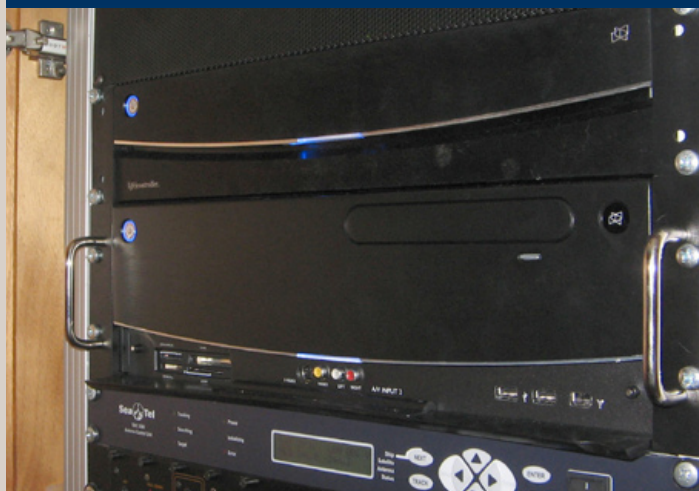
Equipment rack includes a Life|media Digital Media Server and Life|controller Automation Server for audio and entertainment.
